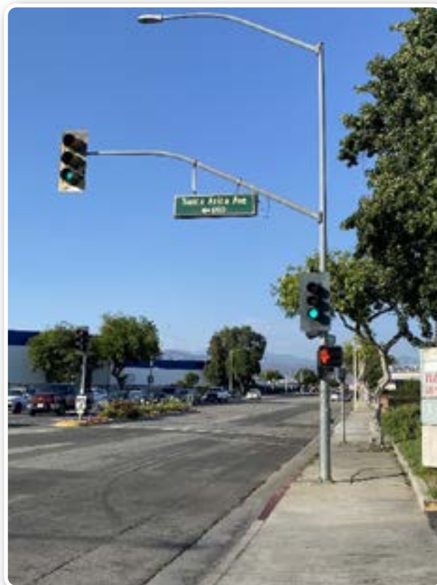
Figure 3: Faded backplate on mast arm, existing 8" bulb vehicle head on pole
