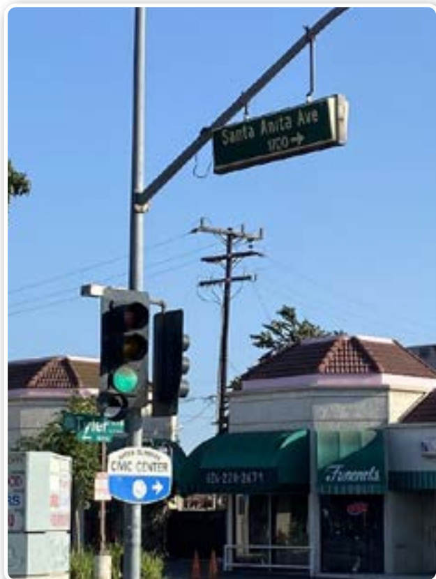
Figure 2: Existing 12" vehicle head with broken bulb hood
